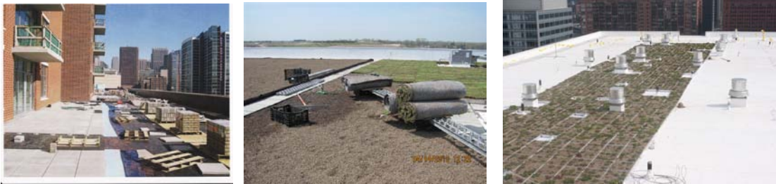
“Where are the roofers?” Wind, Rain, Strikes, have caused the ‘Summer from Hell’
